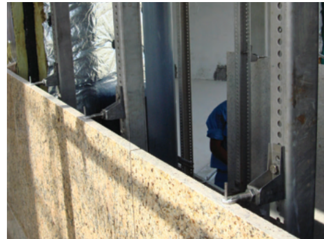
Stone installation made on to stainless steel channel system. T31 undercut bolt is used with specially designed anchors. T31 bolt is fastened on to the anchor using contra nuts.
