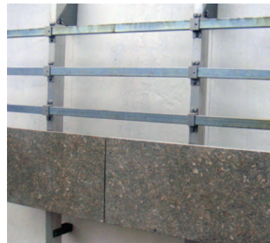
Stone installation made on to stainless steel channel system. T31 undercut bolt is used with specially designed anchors. T31 bolt is fastened on to the anchor using contra nuts.
